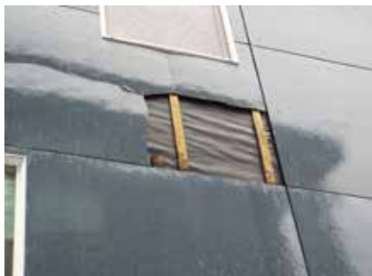
Figure 14: Fiber cement product failure
