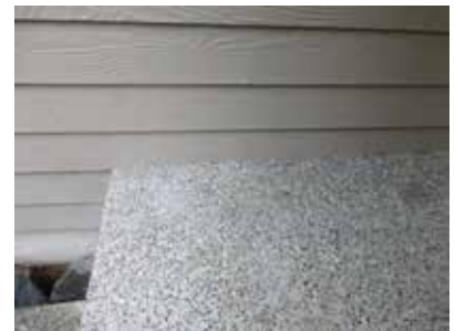
Figure 10: Concrete over siding
