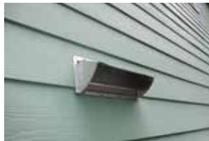
Figure 4: Kitchen Fan Vent
